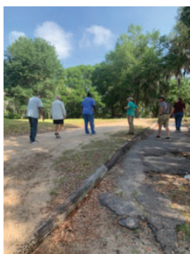
Georgetown Commissioners view the damaged road on Sandy Island in need of repair.
