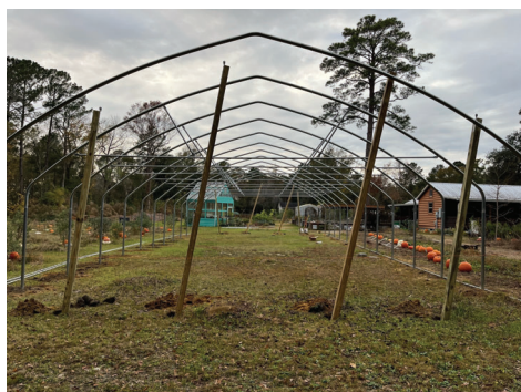
Initial steps of high tunnel installation in Awendaw, SC. Setting posts and framework.
