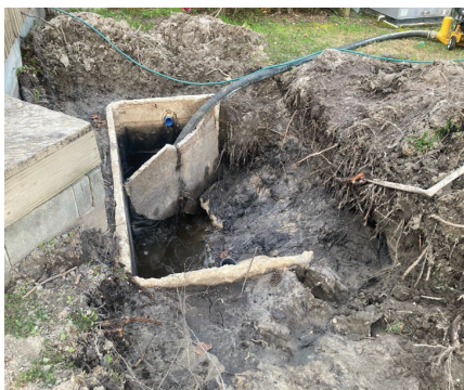
Before water quality project funding assisted in fixing a failing septic tank system.
