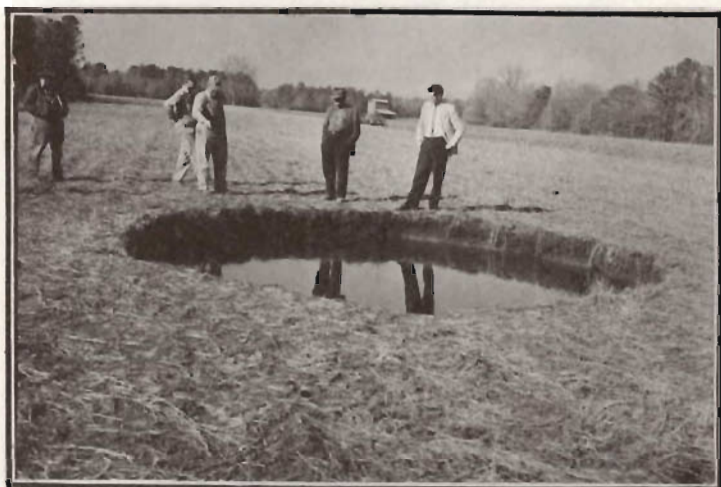
A. SINKHOLE AS IT APPEARED IN JANUARY 1962.
