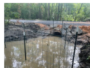
A beaver management project was conducted to show the benefits of using the excluders constructed above to prevent beaver access to the pipes.
