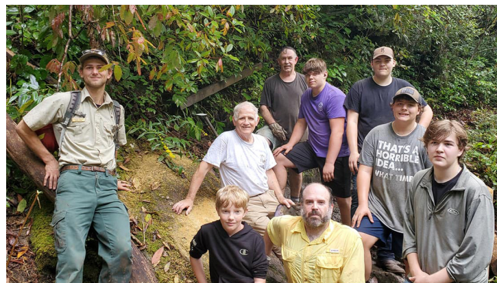
Ethan Sexton helped rebuild an eroded section of the Foothills Trail along the Chattooga as part of his 2021 Eagle Scout project.
