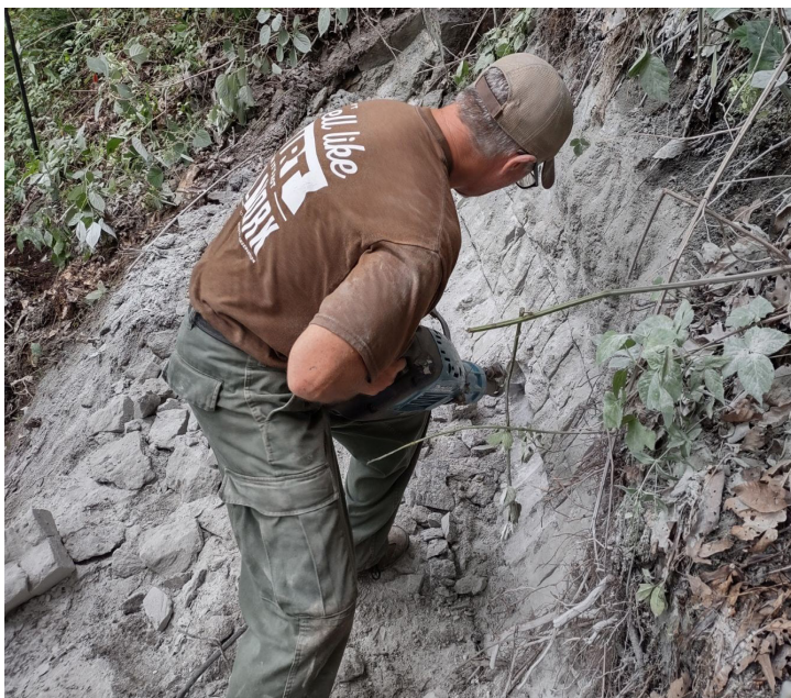
Kevin Evans gets low and stable as he works to drill into granitic gneiss while working on a footpath for the Palmetto Trail.
