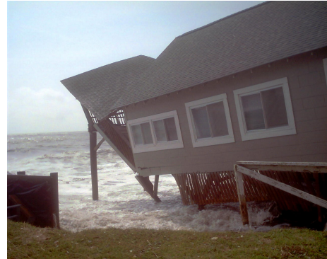
House on Edisto Beach collapses due to coastal flooding from TS Tammy (Photo by Delaine McJunkin)
