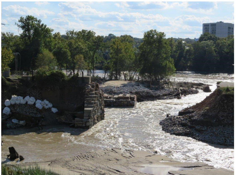
Columbia Canal Breach
