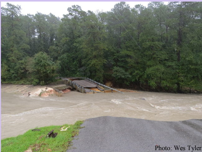
Cary Lake Dam Failure at Skii Lane
